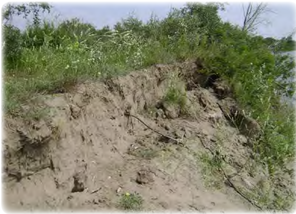
Finlayson Island Bank Erosion (credit: AECOM)
